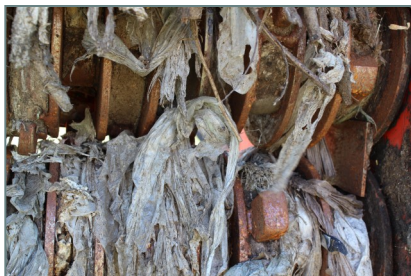
Compostable bags and paper cups stuck in the grinding equipment at the LRCRC.
